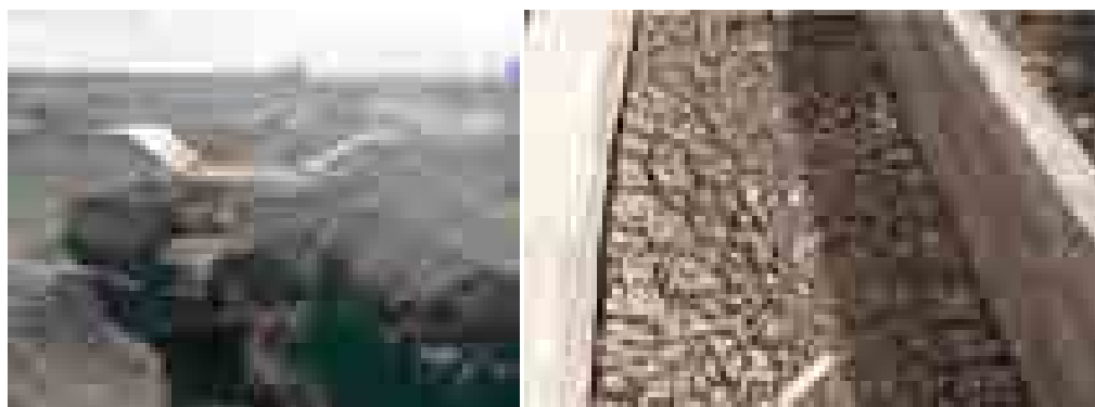
Figure 2.14. Damaged flume structure and silt-filled canal.
